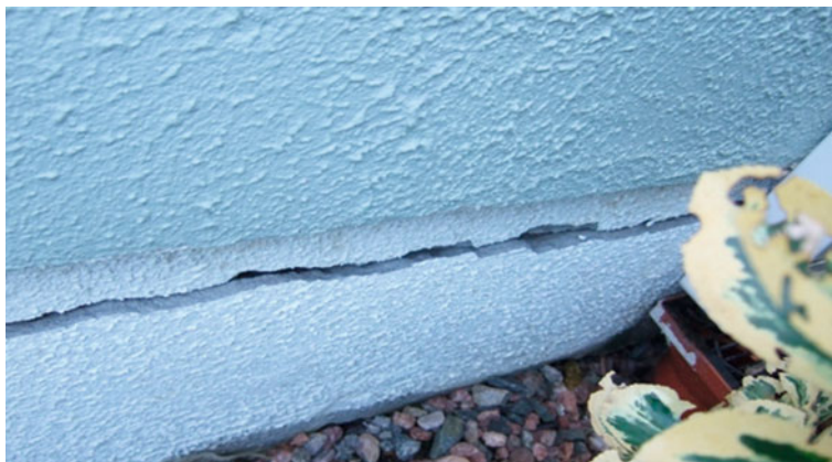
Fig. 18 Cracking and displacement of external wall (plinth)
