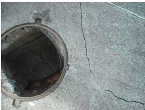
Fig. 21 Pavement cracking near manhole
