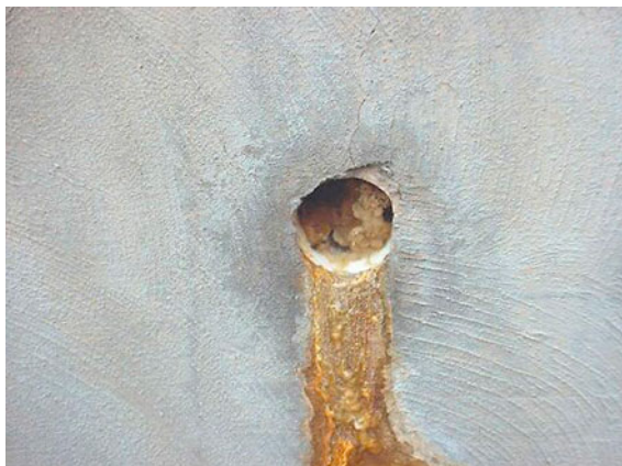
Fig. 20 Sulphate precipitates around drain pipe (2000)
