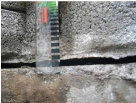
Fig. 22 12 mm gap near top of manhole
