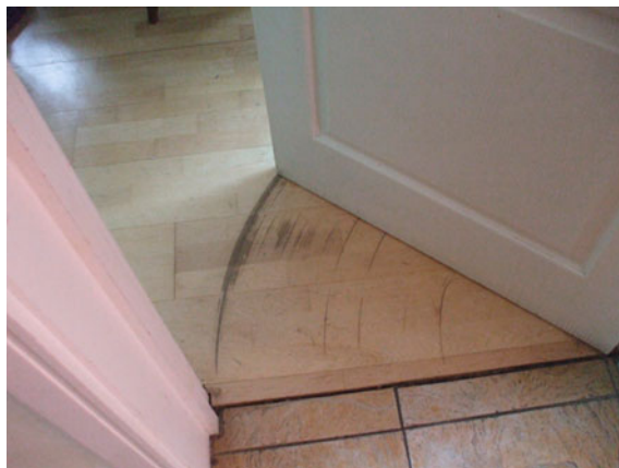
Fig. 14 Bottom of door binding against floor
