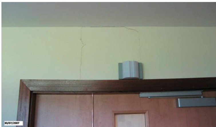
Fig. 15 Top of door binding against architrave
