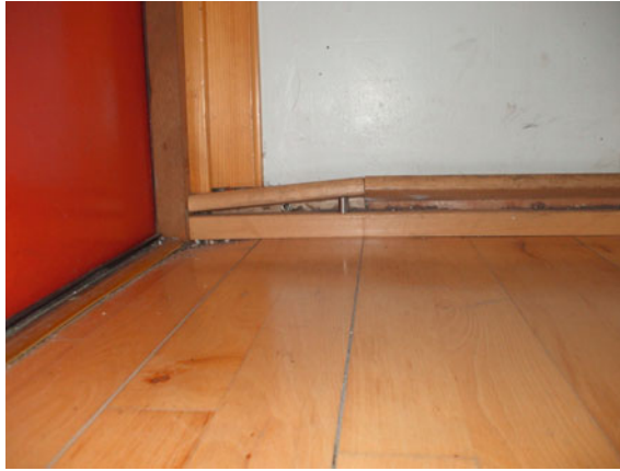
Fig. 12 Displacement of timber skirting
